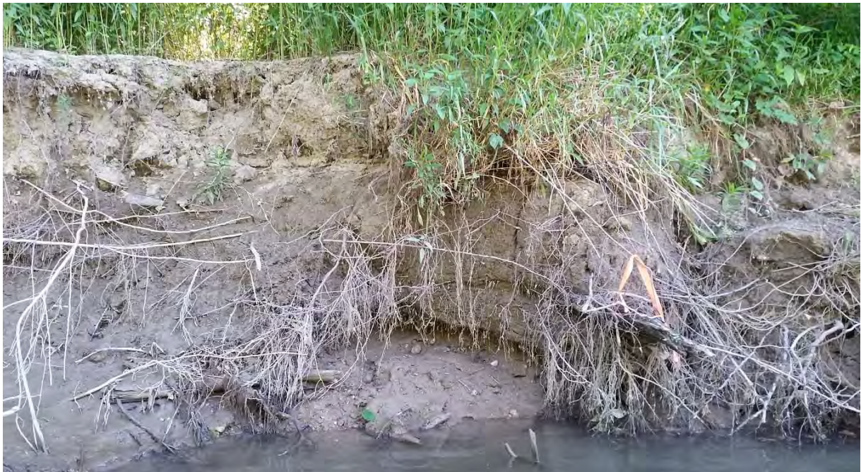
Photo 2: Erosion at the FEH site (Note eroded slope and lack of vegetation)
