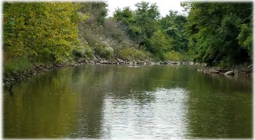
Figure 2: Failed Streambank above Revetment at FEH Site
