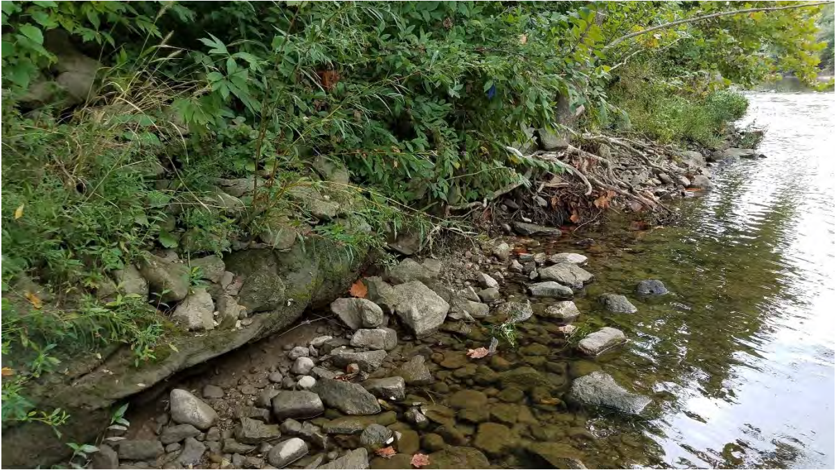
Photo 5: Exposed erosion control blanket and riprap (east bank)
