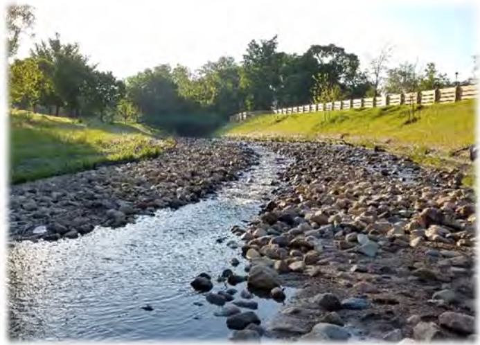
Figure 9: Armored Channel in Indianapolis, IN
