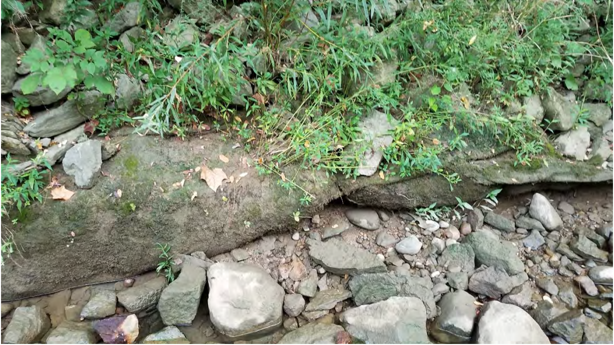
Photo 7: Exposed erosion control blanket (east bank)
